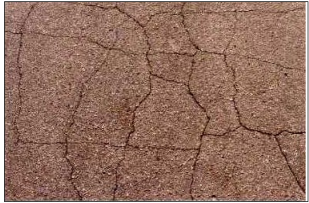
Condition 5 – Very Poor
